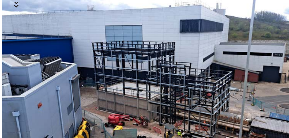
Latest progress at the new HRPD-X facility, ISIS Neutron and Muon Source, Rutherford Appleton Laboratory - where the steel frame is now in place
